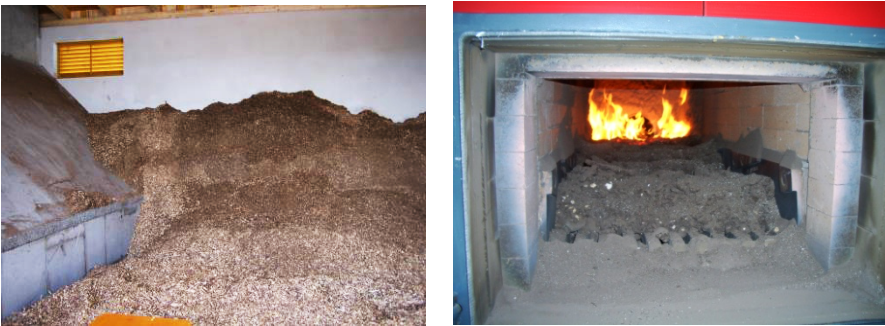
Figure 63. Wood chip storage and furnace of heat plant Hofstetten-Grünau (BIOENERGY2020+)
