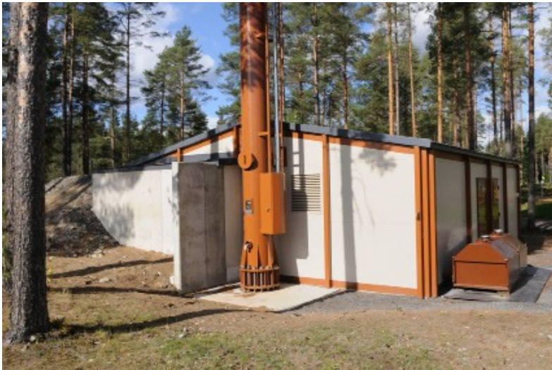
Figure 73. Maxicont 250 heating container (Megakone Oy)
